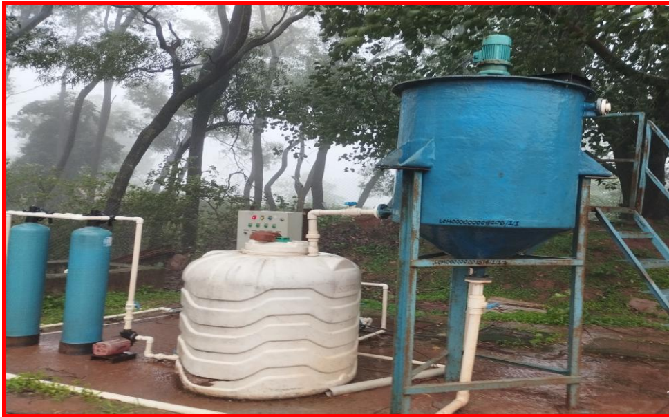
Effluent Treatment Plant
