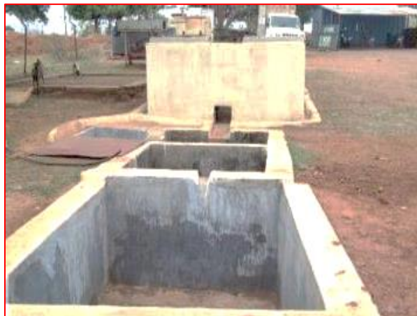
Washing Ramp and Oil & Grease Trap
