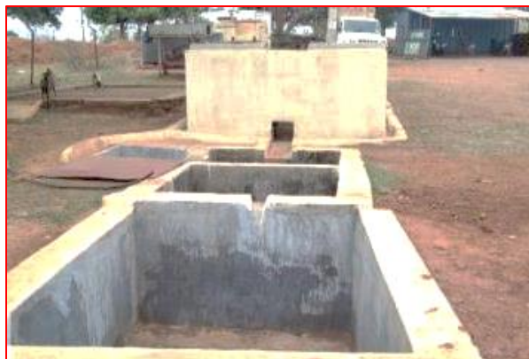
Washing Ramp and Oil & Grease Trap
