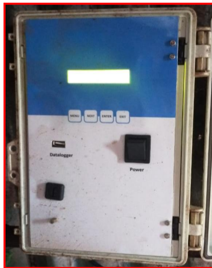
Piezometer at Kujam I Mine
