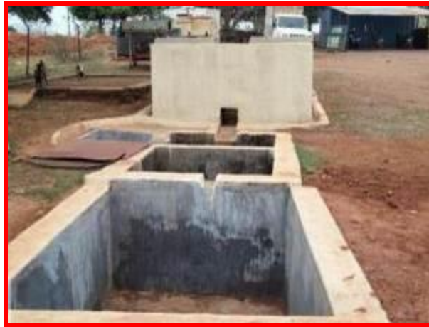
Washing Ramp with Oil & Grease Trap
