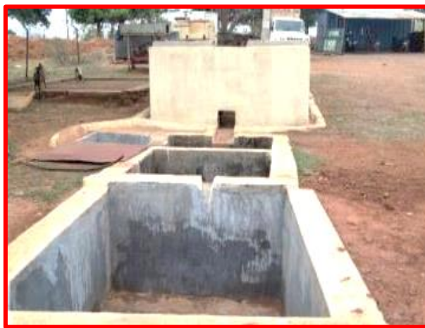
Washing Ramp and Oil and Grease Trap
