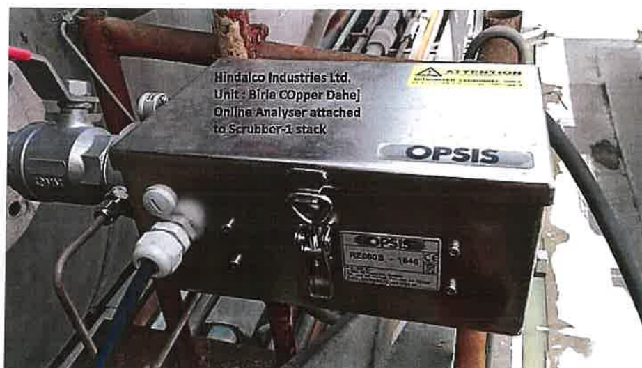
CEMS at Smelter-1
