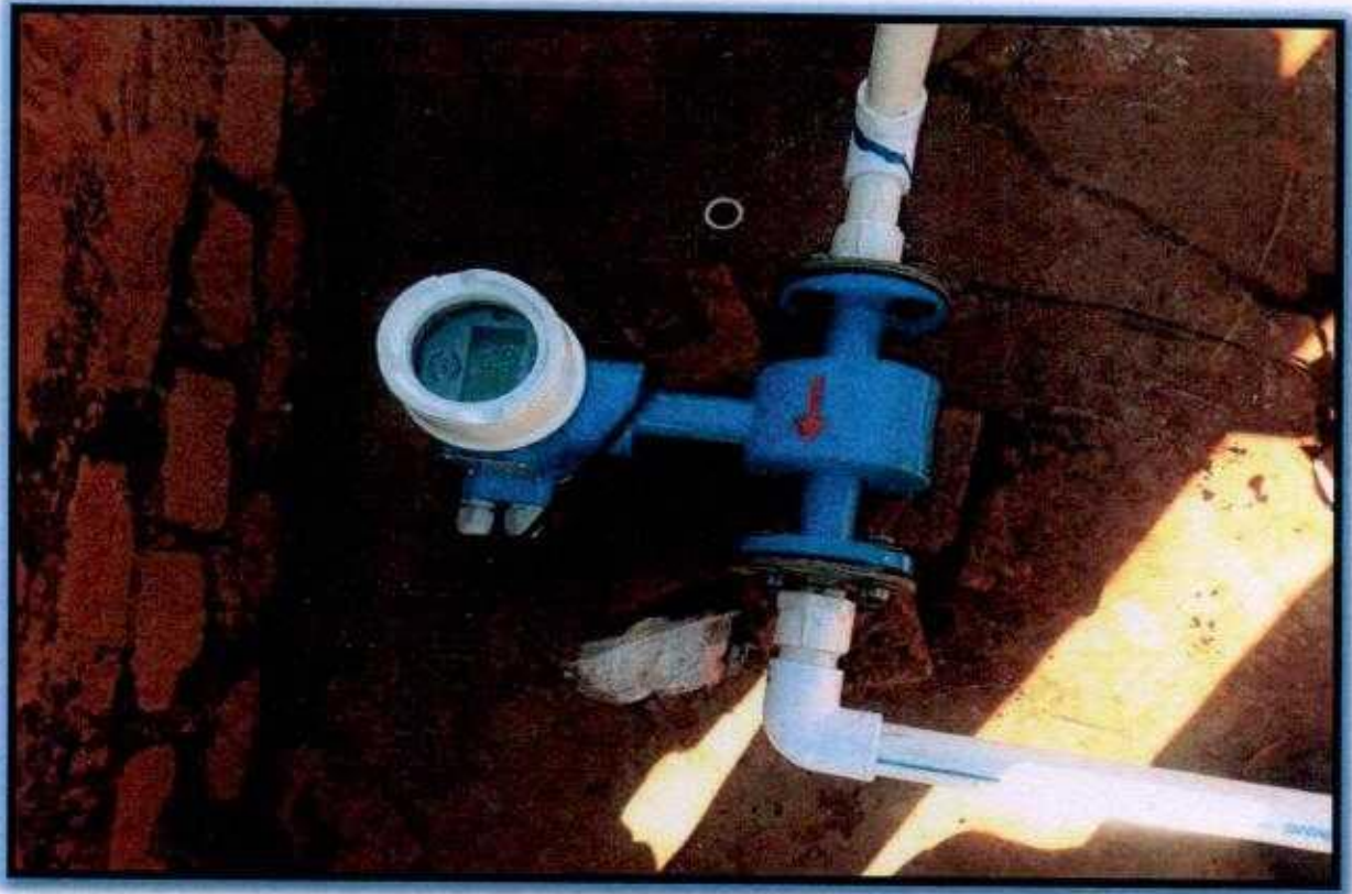
View of Digital Water Meter Installed in the Lease area
