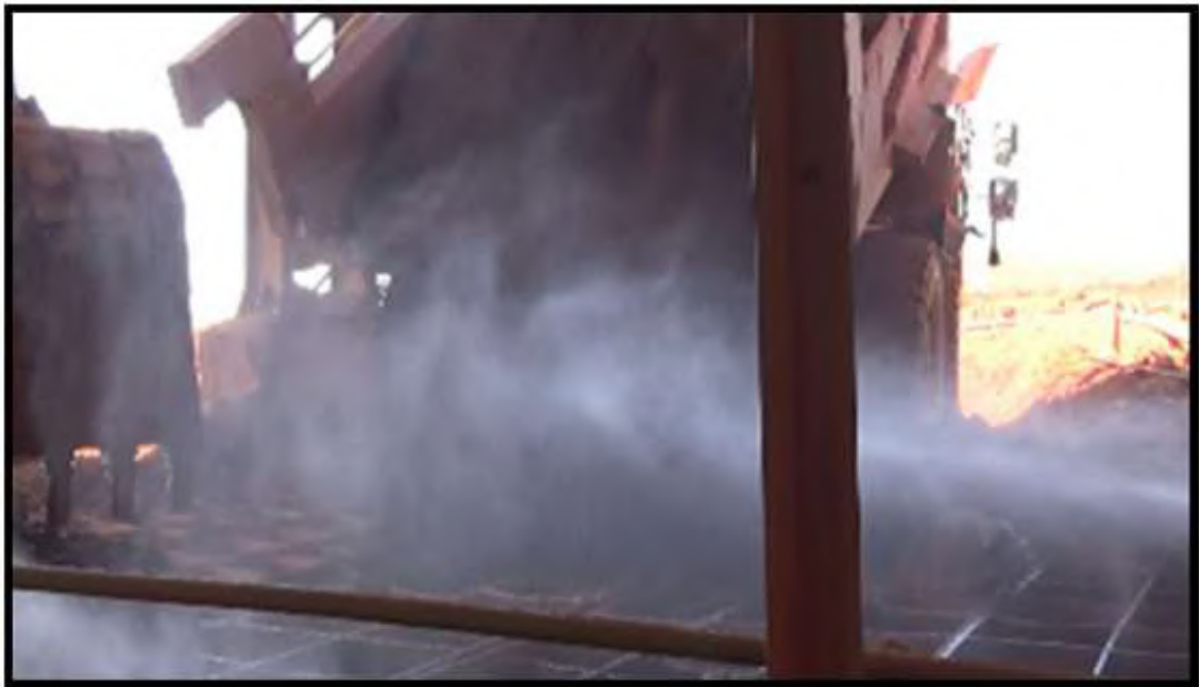
PHOTO 13: Showing Dry fog system in Fixed Crushing plant
