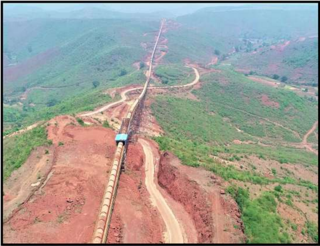
PHOTO 12: Showing Covered Long distance Conveyor
