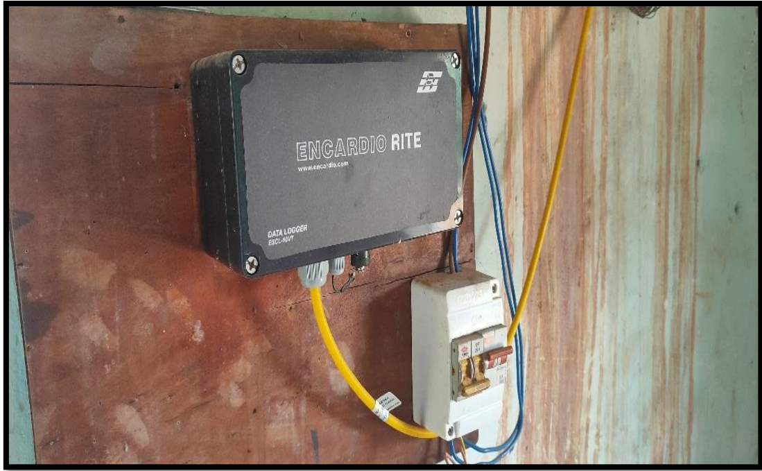
Piezometer installed in our Lease area
