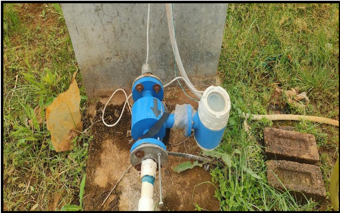
Water Meter - Telemetry
