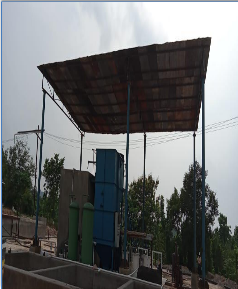
ETP of capacity 50 m 3 /day at Bankheta – GP IV/4 Coal Mine
