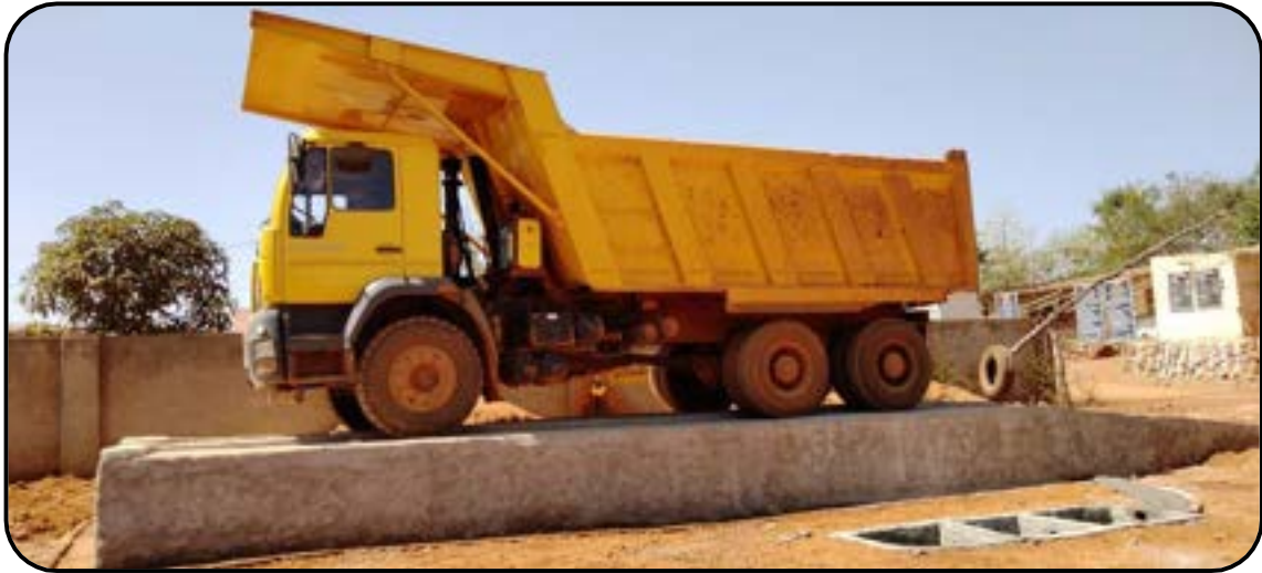
Pic: Washing platform and oil & grease trap.
